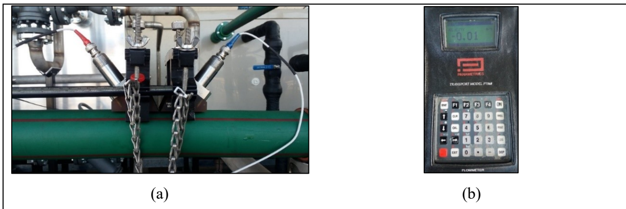
Figure 19 – Photographs of the applied flowmeter sensors (a) and the GE Panametrics PT868 signal acquisition system (b).
