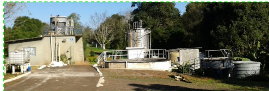
Swine wastewater treatment plant - SWTP
