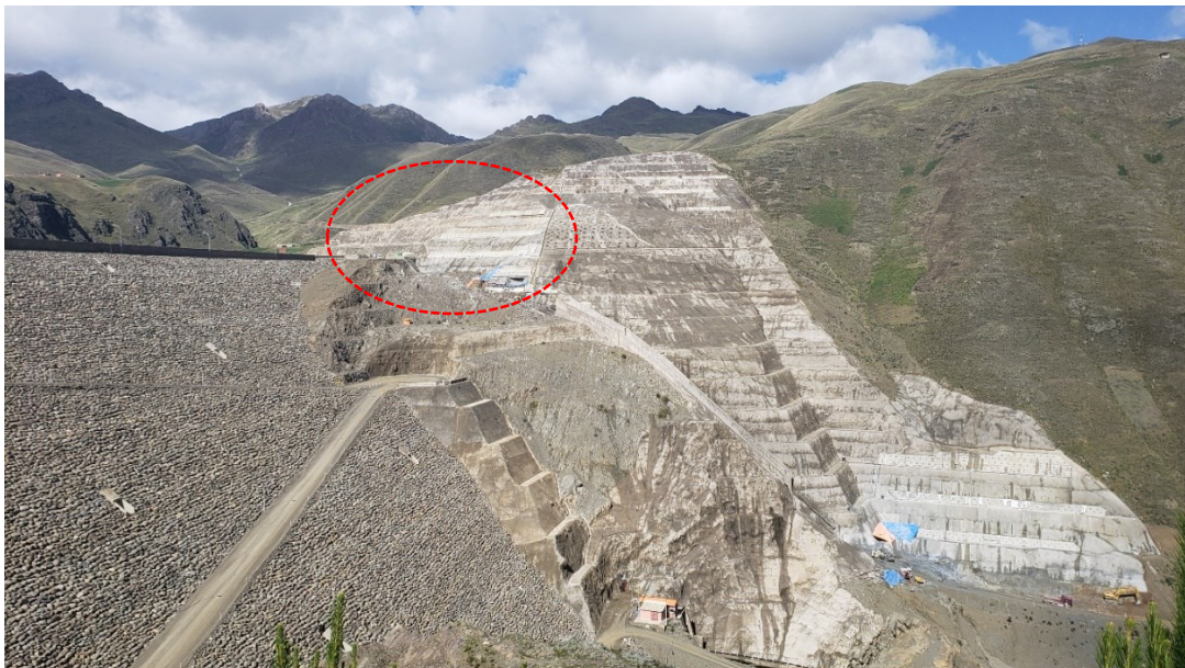
Fig. 2. General view of the Misticuni Dam and the spillway excavation slope. The red circle shows the location of the excavation slope.
