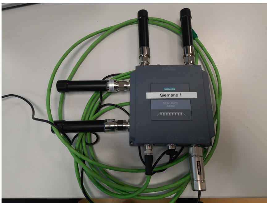
Figure 13 – Siemens Scalance M800 router. Source: Author.
