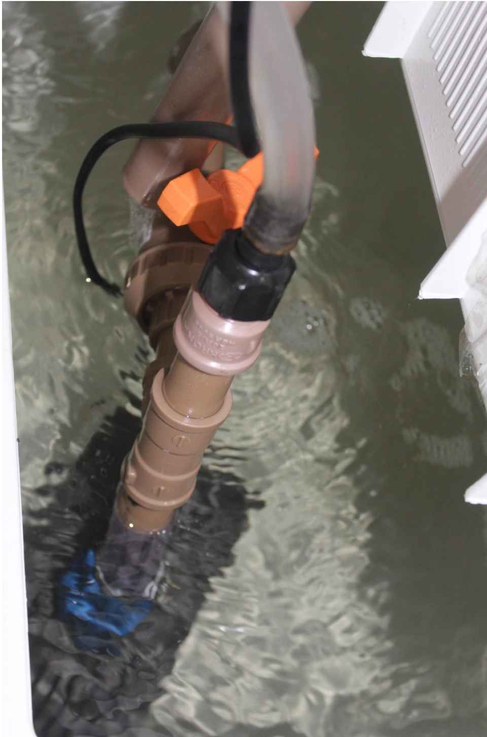
Apêndice I - Water recirculation pump. Photo by Marcelo Santana
