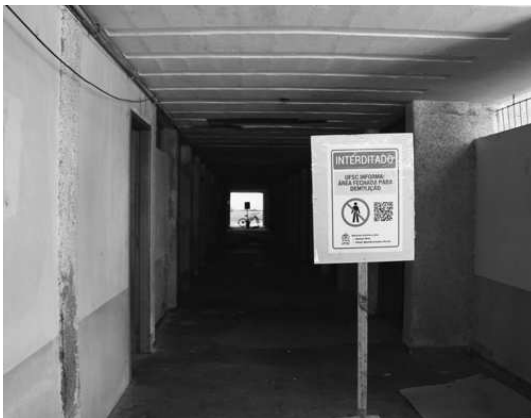
Figure 125. General view of the low-rise buildings surrounding the EFI. The sign warns users that part of the building has already been cordoned off for demolition. 2025. Source: UFSC.
