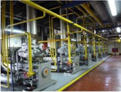
Figure 11: Engine room, where are all the electric motors and emergency generator system.
